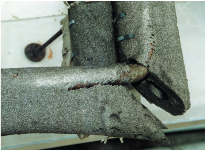
Figure 4.53 Damaged thermal insulation
