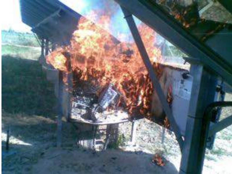
Improper design and installation can cause fire in a PV system
