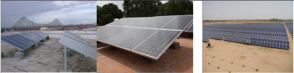
Examples of grid connected PV systems: Rooftop distributed systems and MW scale project
