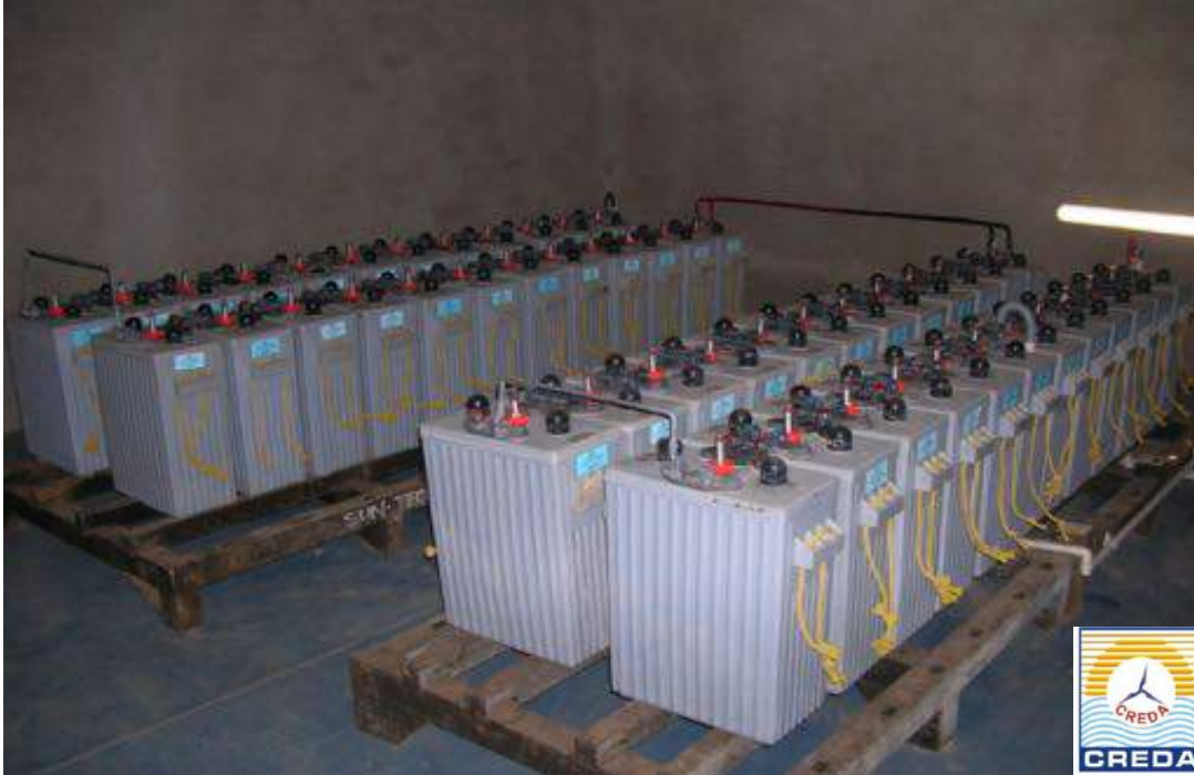
Location of battery bank in a separate well ventilated room
