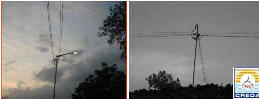
Power distribution lines connecting the load centres
