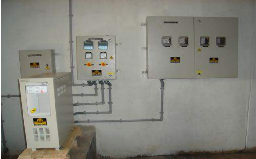
Example of control centre wiring
