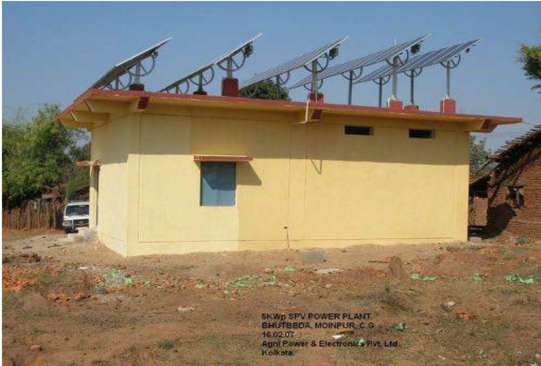
Example of array installed on a RCC roof of the control room
