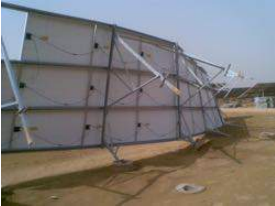
Poor quality structure and foundation
