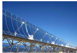
Concentrated Solar Power (CSP)
