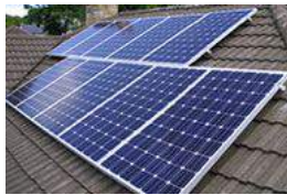
Solar Photovoltaic (PV) Systems
