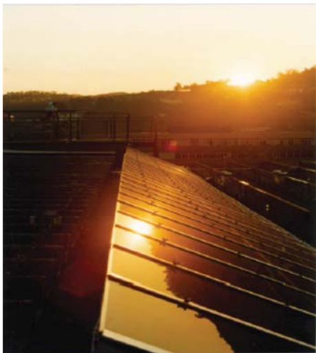
Fig. 7.9 Lateral view of the 2 kWp a-Si thin-film PV installation in Florianópolis, Brazil (with permission [Rüther-1998]).
