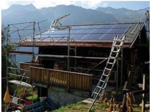
Fig. 7.4 PV roof integration Mungg in Bellwald (1600 m), Switzerland.
