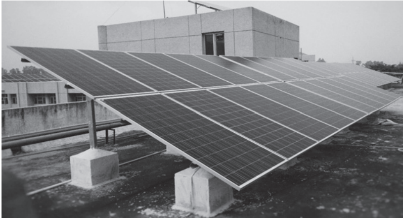
FIGURE 11.21 5 kW p PV system installed on the rooftop of the EEU laboratory, Delhi Technological University, Delhi, India.
