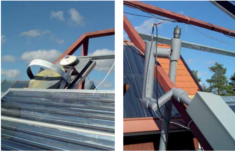
Figure 3.7 The pyranometer mounted in the collector plane (to the left) and the inlet piping with an air trap and a vent (to the right).
