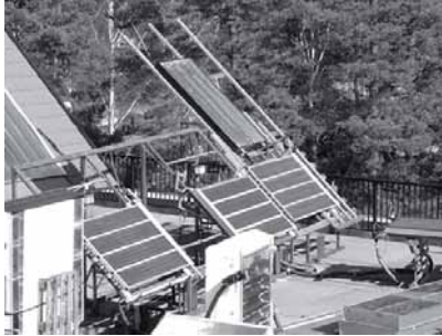
Figure 5. The collectors mounted outdoors for long-term evaluation in Älvkarleby, Sweden.
