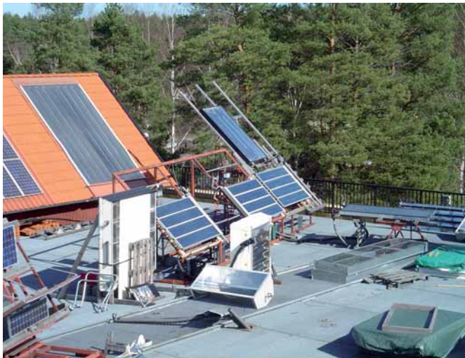
Figure 3.6 The collectors mounted outdoors at the Älvkarleby test facility.
