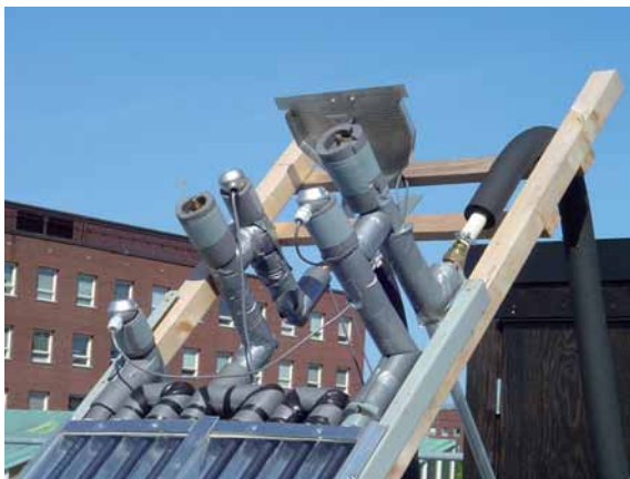
Figure 3.2 Insulated air vents and Pt 100 sensors on the collector inlet and outlet.
