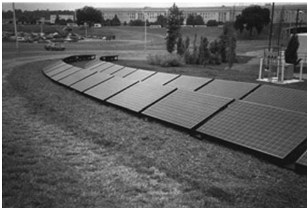
FIGURE 5.8 Solar Module System: Supplying Power to Pentagon
