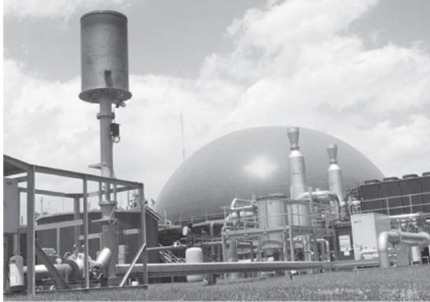
The Laikipia anaerobic digester.
