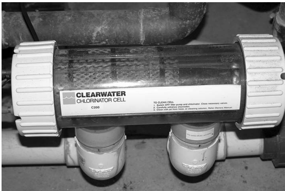
Figure 6.2 Photo of Clearwater solar powered pool chlorinator.
