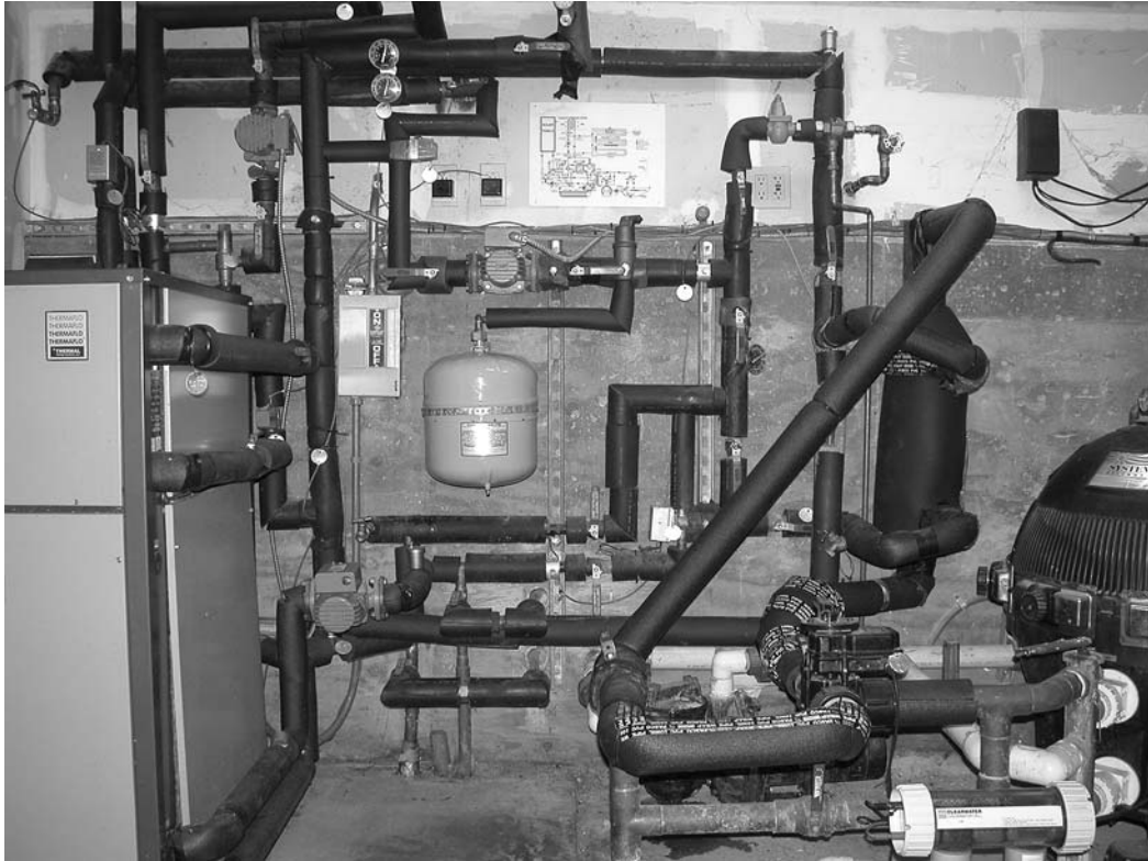
Figure 7.8 Photograph showing the solar piping/control system.
