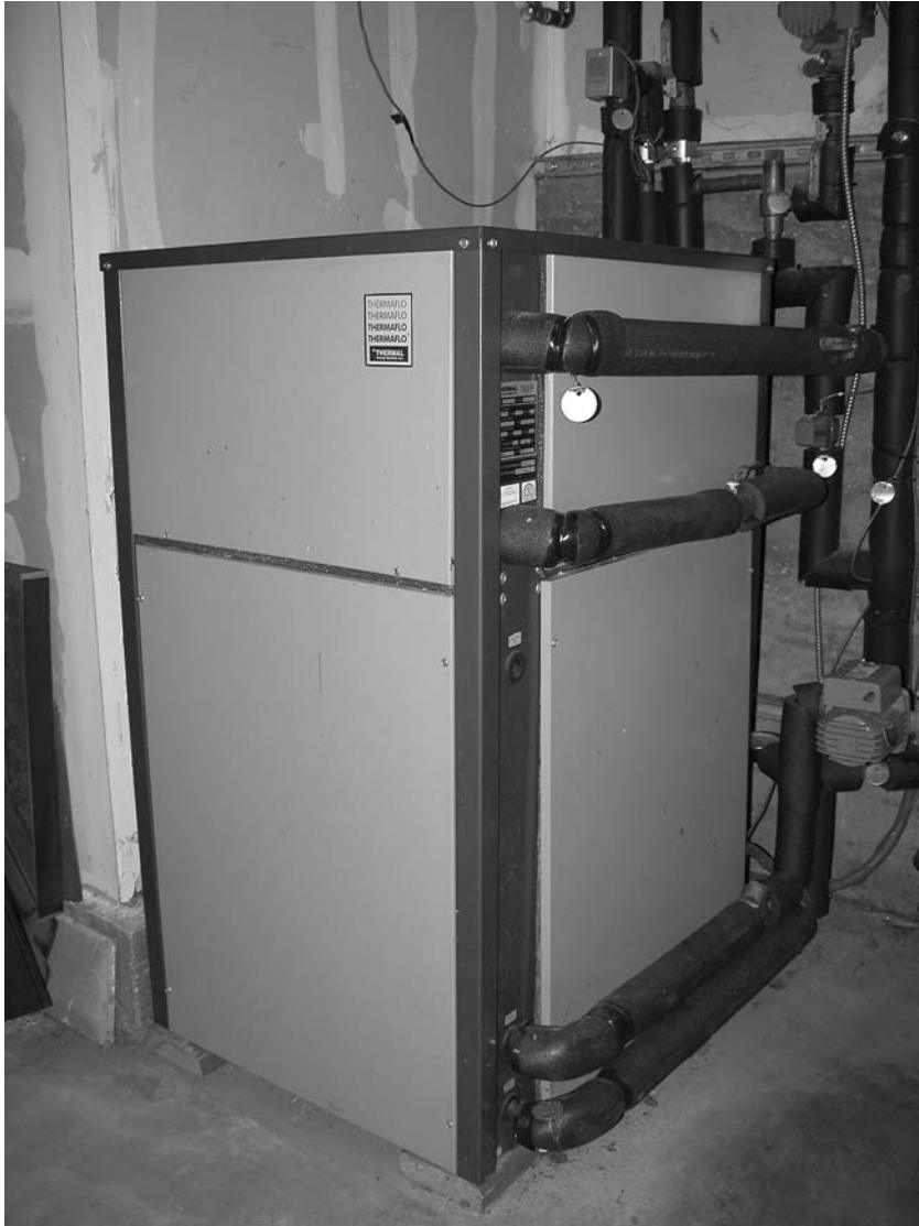
Figure 7.6 Photograph of Berkeley house geothermal heat pump.
