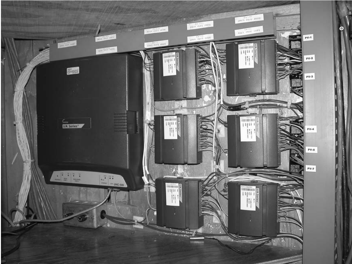
Figure 7.11 Photograph showing control closet hardware.
