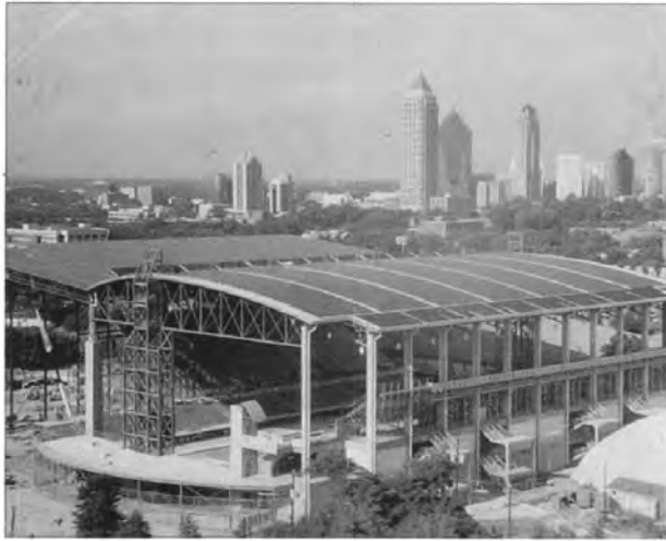
FIGURE 3-8 Roof (pv) of Atlanta's Aquatic Center with 345 kW grid-connected power system. (Source: Georgia Institute of Technology. With permission.)
