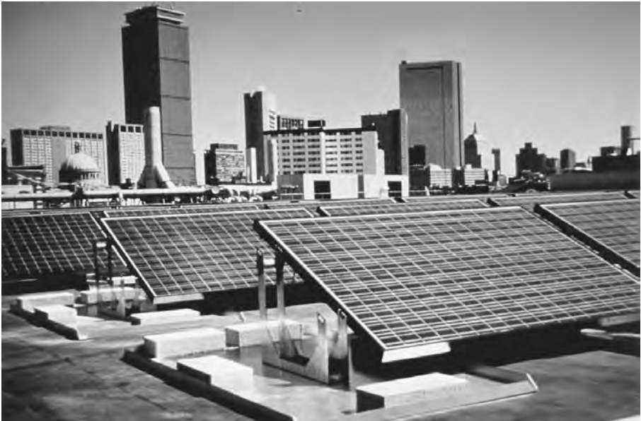
FIGURE 13-2 18 kW grid-connected pv system on the Northeastern University Student Center in Boston, MA. (Source: ASE Americas, Billerica, Massachusetts. With permission.)
