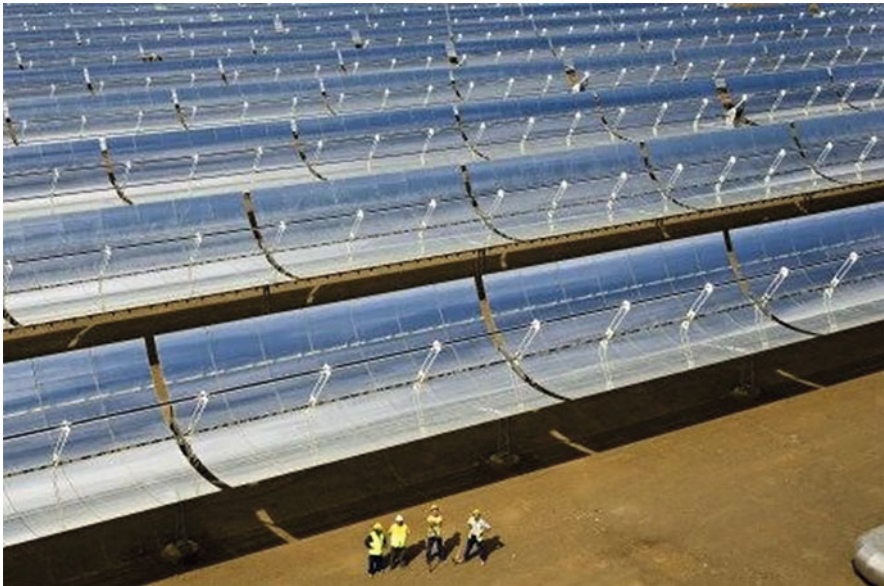
Fig. 4.6 Typical parabolic-trough collector solar field
