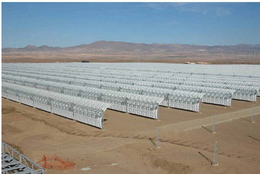
Fig. 2.15 Solar field of the Andasol-1 plant
